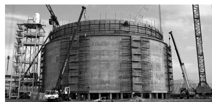
Widok stokażu amoniaku View of ammonia storage tank
